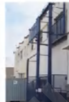
Mechanical freight elevator
